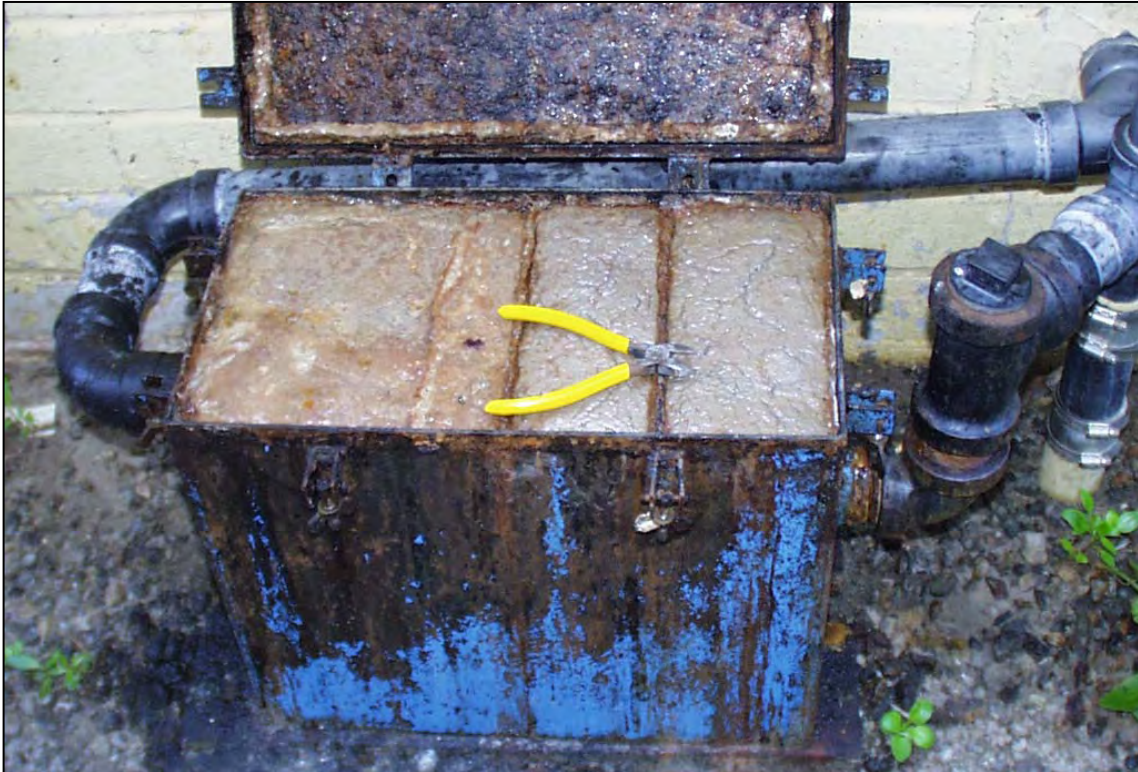
FIGURE 6-19 Passive Grease Trap requiring maintenance (Courtesy of Monterey Regional Water Pollution Control Agency)
