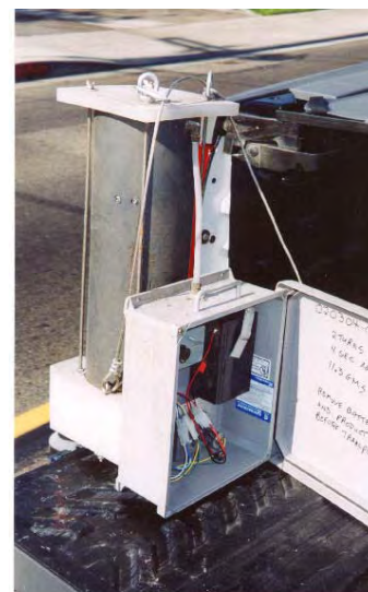
4. Control panel opened to record or adjust feeder pumping rate.
