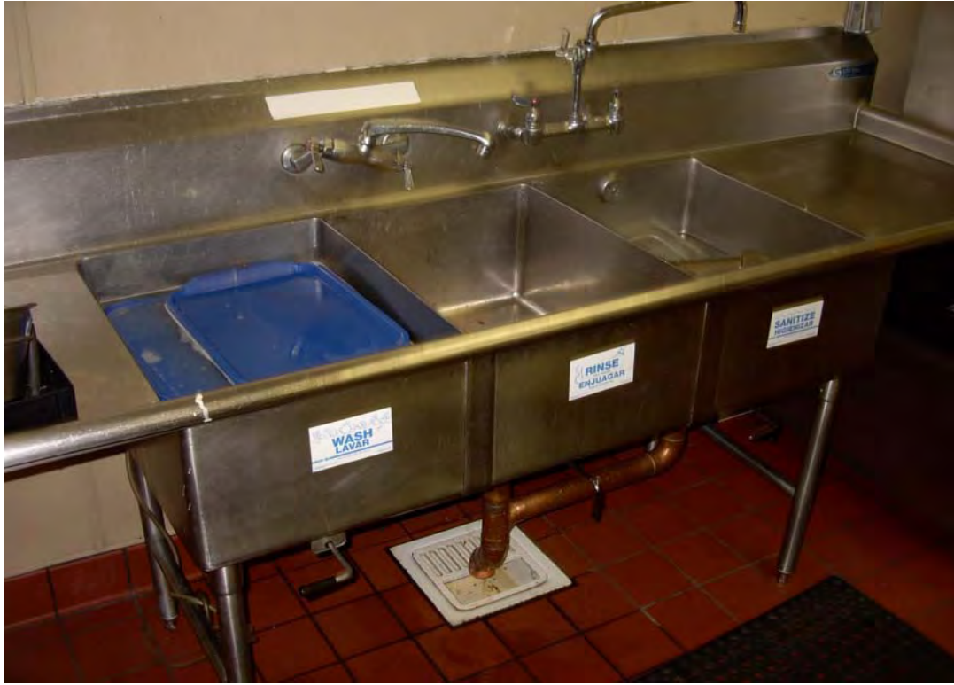
FIGURE 6-2 A Three-Compartment Sink Discharging to a Floor Sink with a Drain Screen
