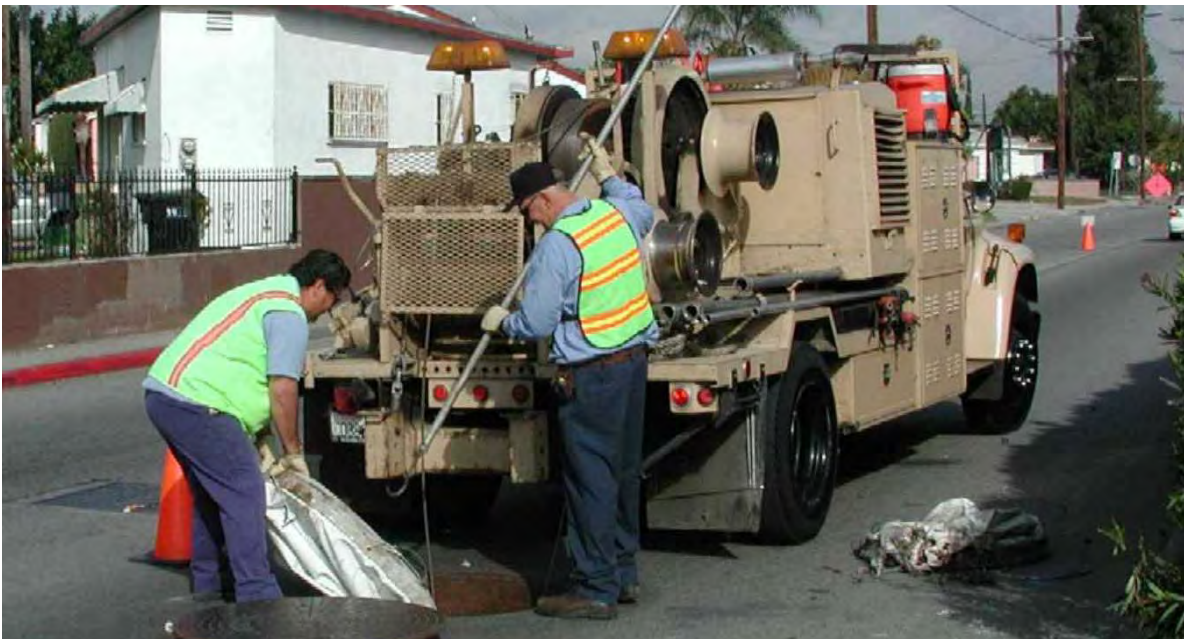
FIGURE 6-7 Sewer Line Cleaning (Courtesy of County Sanitation Districts of Los Angeles County)
