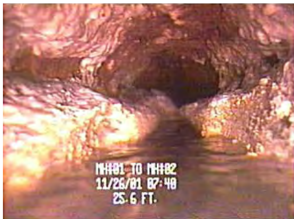
1. Video image before Ennix pilot test, showing grease build-up.
