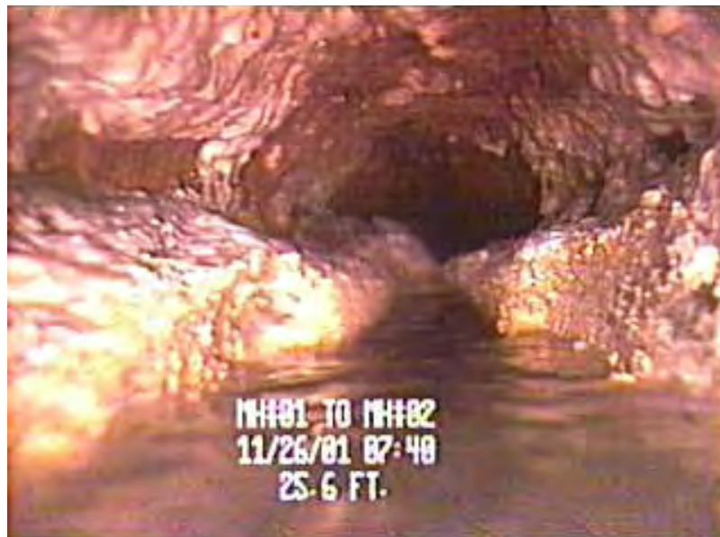
FIGURE 6-8 CCTV Inspection of sewer line with grease build-up
