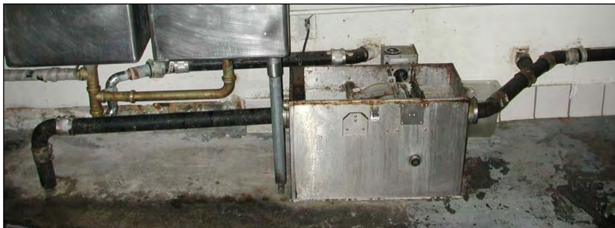
FIGURE 6-21 Automatic Grease Trap installed under a sink – lid removed for photo (Courtesy of County Sanitation Districts of Los Angeles County)
