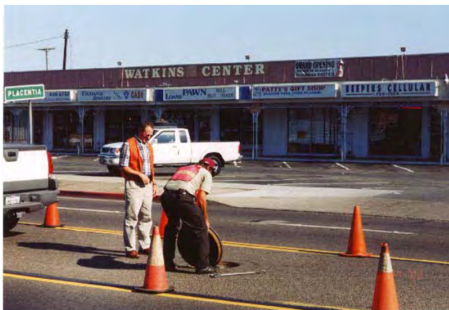
1. Feeder location on 19 th street.
