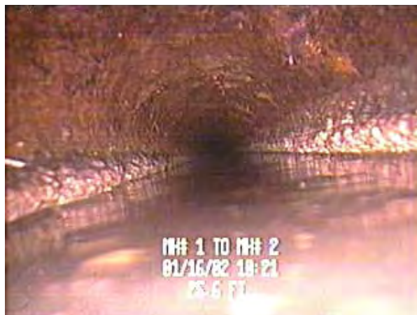
2. Video image after 50 days of Ennix pilot test, without sewer line cleaning.
