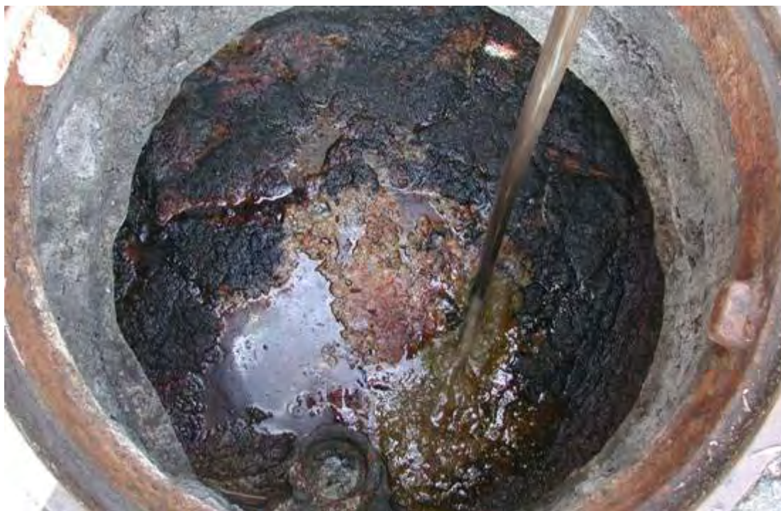
FIGURE 6-14 Interceptor – Solids and grease accumulation being measured with a clear pipe device called a “Sludge-Judge” (Courtesy of County Sanitation Districts of Los Angeles County)
