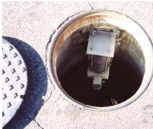
2. Feeder mounted on ladder under the manhole.
