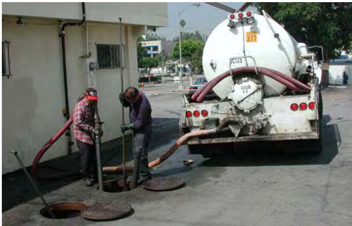
FIGURE 6-13 Interceptor Maintenance – Interceptor being cleaned and pumped (Courtesy of County Sanitation Districts of Los Angeles County)
