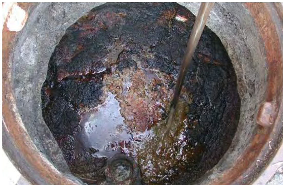
FIGURE 6-26 Interceptor Monitoring – Solids and grease accumulation being measured with a clear pipe device called a “Sludge Judge” (Courtesy of County Sanitation Districts of Los Angeles County)
