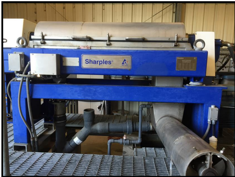
Centrifuge Unit at Rancho Santa FE WRF
