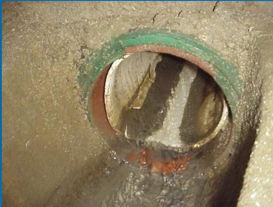
End seal not installed
