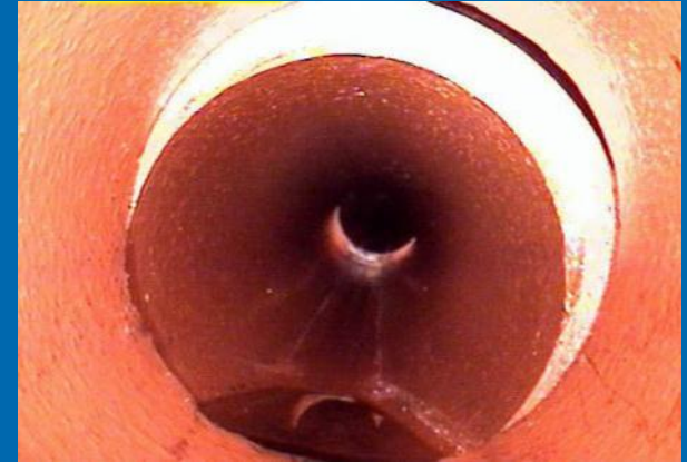
Severe Offsets over \frac{3}{4} "
