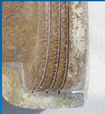
Bottom of pipe joint No grout
